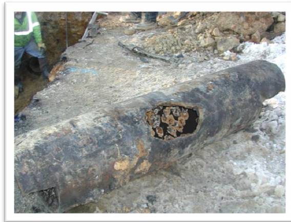
The 16" cast iron pipe from North Main Street showing the hole that blew out.
